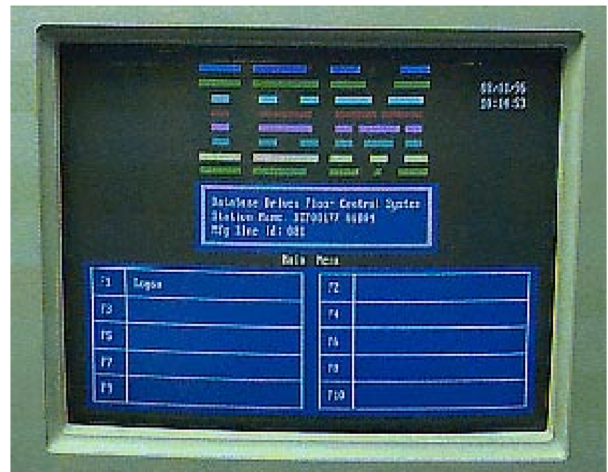
Data Base Floor Control System
