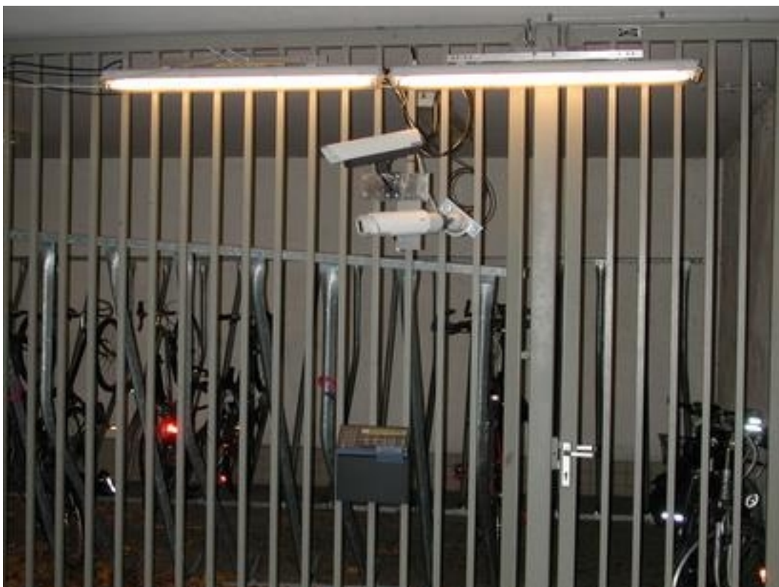
Figure 119: the camera installation including the additional lighting
