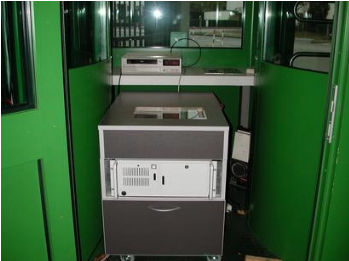
Figure 120: computer installation in the booth to the right
