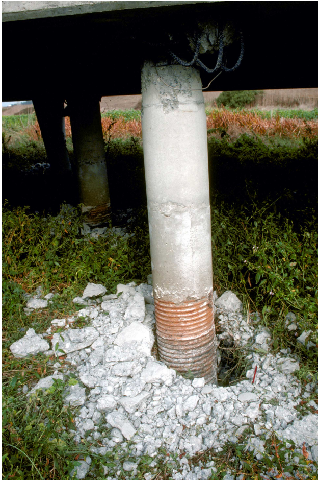
98. Support column of bridge across Struve Slough, Highway 1. Enlargement of hole where support enters the ground is an effect of lateral shaking, which caused the concrete to break up where the column joined the bridge and was instrumental in the roadbed collapse. [H.G. Wilshire, U.S. Geological Survey]
