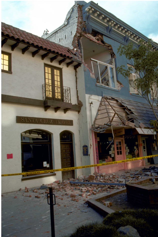
78. Storefront damage, Pacific Garden Mall. [C.E. Meyer, U.S. Geological Survey]
