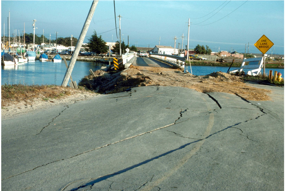
101. Ground cracking and differential settlement due to liquefaction of beach and Salinas River deposits damaged approach and abutment of bridge linking Moss Landing spit to the mainland, near Moss Landing Marine Laboratory. [J.C. Tinsley, U.S. Geological Survey]
