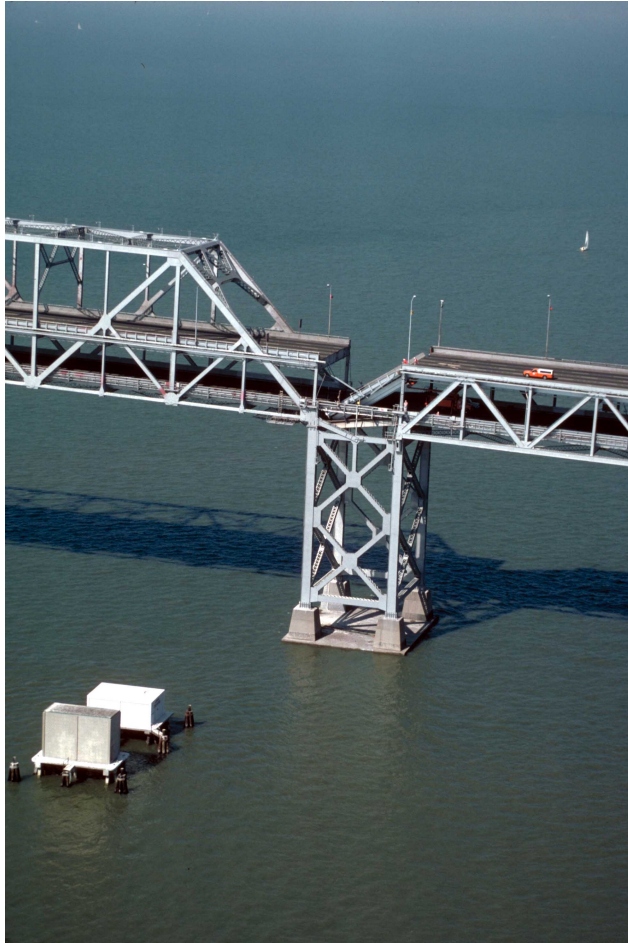
15. Aerial view of roadbed collapse near the interface of the cantilever and truss sections of the San Francisco-Oakland Bay Bridge. View northwestward. [C.E. Meyer, U.S. Geological Survey]
