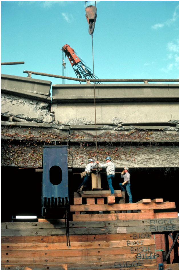
28. Temporary support structures emplaced to prevent further collapse, Cypress viaduct. [H.G. Wilshire, U.S. Geological Survey]
