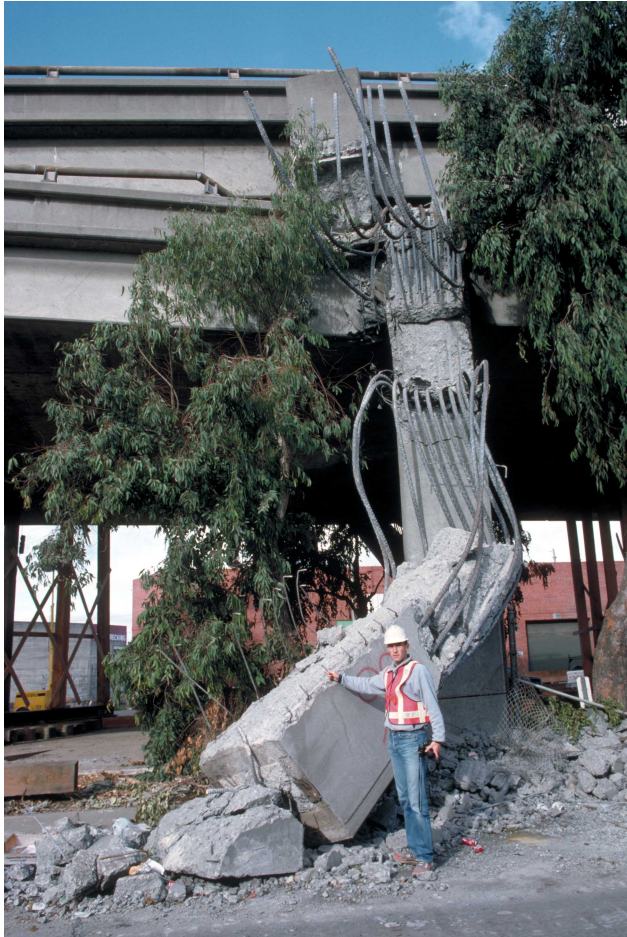
23. Support-column failure and collapsed upper deck, Cypress viaduct. [H.G. Wilshire, U.S. Geological Survey]
