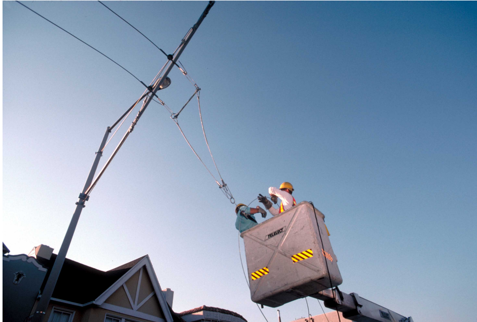
14. Electric wires being removed from unstable towers by city utility workers. Arresting sparks from broken wires was a priority in those areas with broken gas mains. [J.K. Nakata, U.S. Geological Survey]
