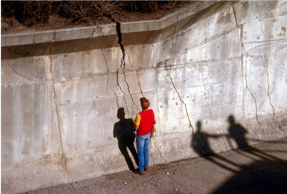
59. Prominent N. 15 o W.-trending extensional cracks up to 12 cm (4.7 in.) wide in concrete spillway to Austrian Dam, north abutment. [G.R. Fisher, U.S. Geological Survey]
