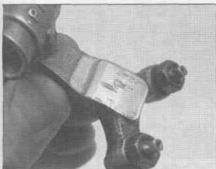
10.38 Inspect the rocker arms, especially the faces that contact the cam lobes, for wear
